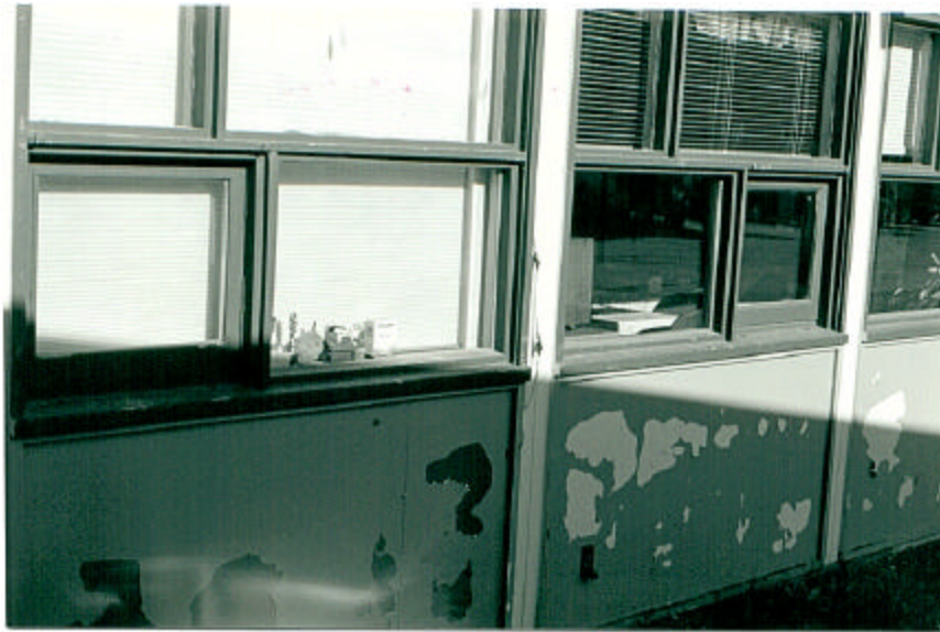
Exterior paint peeling at Rabbit Creek Elementary School.
